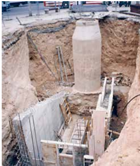
Image 8. Channelling the sewerage network in Calle Fernando Madroñal – Connection with Parque collector
