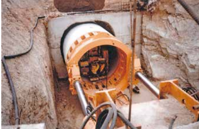
Image 7. Replacing general collector for Section I – Driving Ø2500 under the Gran Vía
